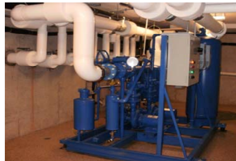
ERG's geothermal system
